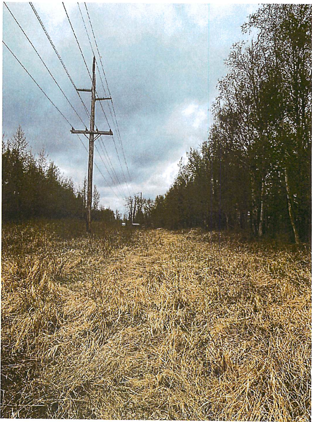
Photo 2 – Powerline on subject property near Bogard Road looking east
