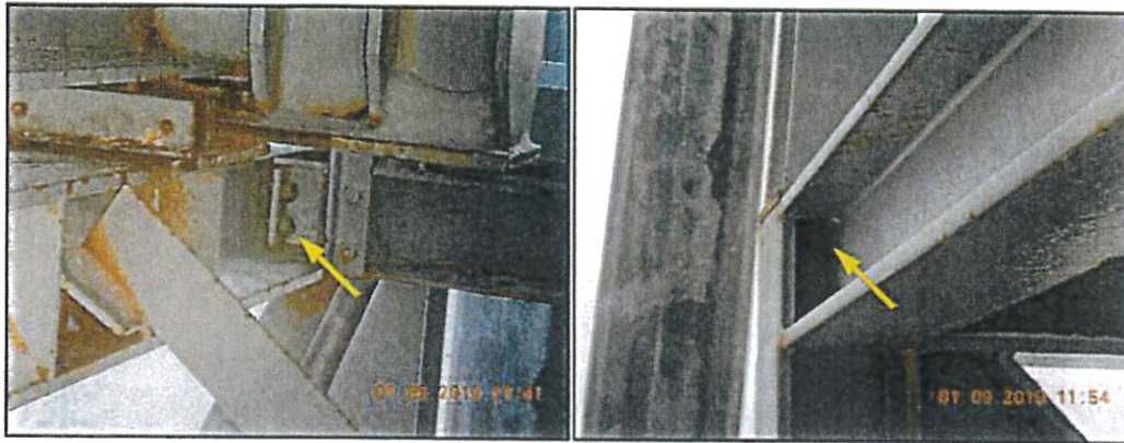
Figure 11: Loose Bolts Around Hopper Framing, typ. (January 2019)
