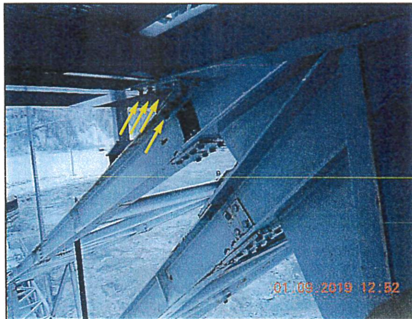
Figure 10: Loose Framing Bolts Near Ship Loader (January 2019)
