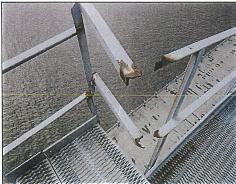
Figure 7: Damaged Catwalk Handrail
