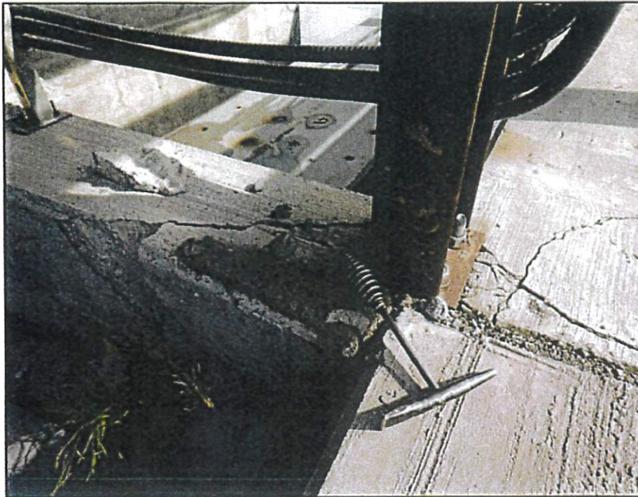
Figure 13: Concrete Damage at Onshore Backwall Conveyor Supports
