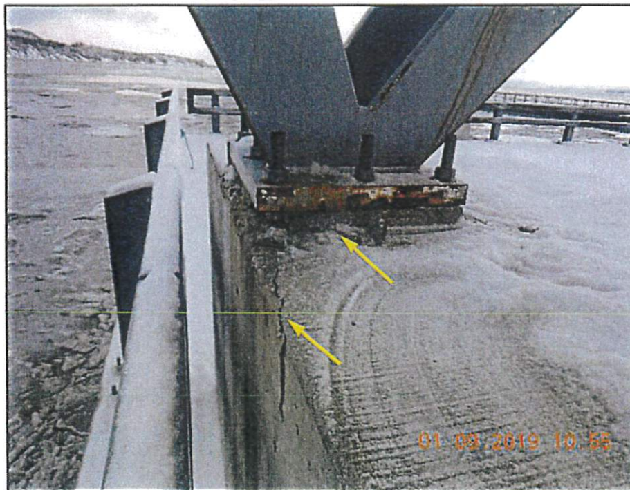
Figure 14: Damaged Grout Pads at Platform Dock Supports, typ. (January 2019)
