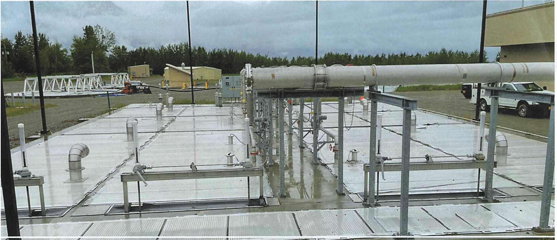
MBBR- Moving Bed Biological Reactor (2018)
